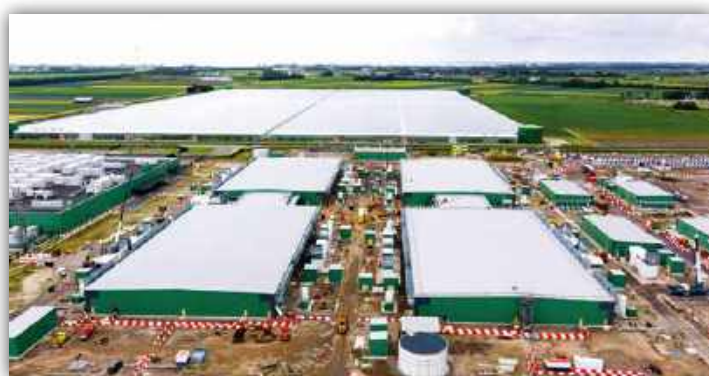
↑ FIGURE 1: AMSTERDAM AZURE DATACENTER
